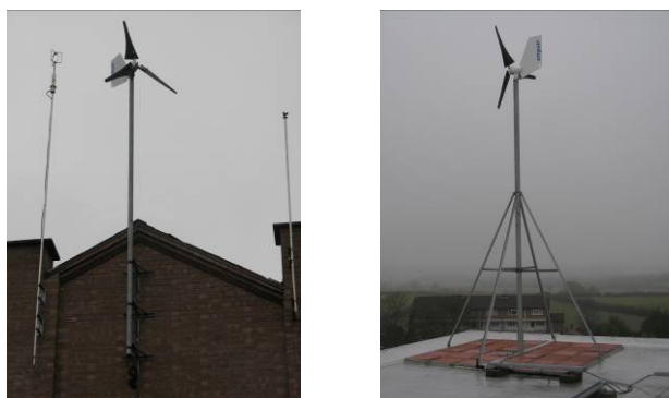
Figure 1: Two building-mounted micro-wind turbines. Left: wall mounted, right: flat roof mounted.
