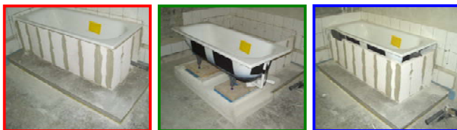
Figure 4: Measured installation noise in an adjoining room (diagonal to installation room) by exciting a bath tub with the EMPA-hammer and different test set-ups. The red curve results from a measurement under practical conditions consisting of a bath tub mounted on a floating floor with enclosure (5 cm aerated concrete). The green curve shows the same bath tub with a very effective structure-borne
