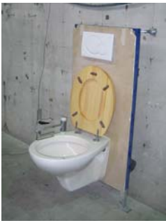
Figure 3: Test set-up, WC-system on the reception plate (corresponding measuring results see figure 2).
