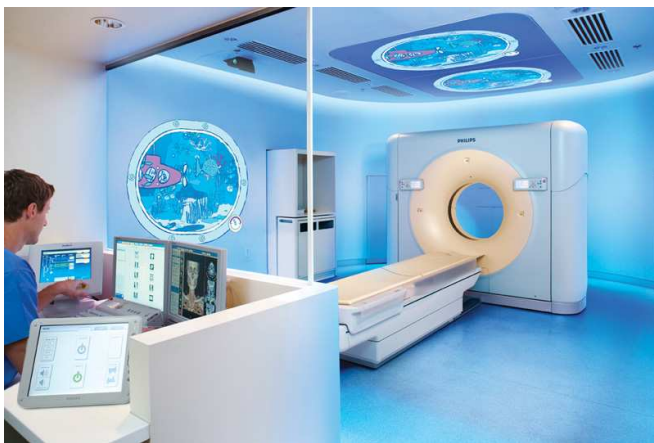
Figure 1: Typical installation of an ambient experience CT scanner, control room view
