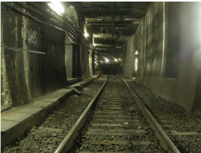
Figure 1: The tunnel before rehabilitation; note the reduced loading gauge and the structural connections of the track to the tunnel walls.
