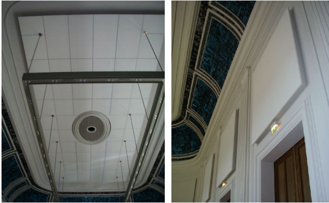
Figure 3: "Aula", Broadband Compact Absorbers at the ceiling behind a fabric lining.
