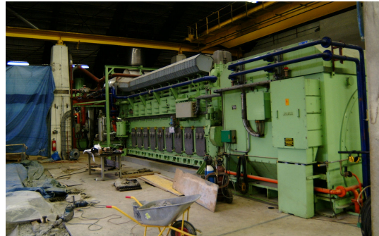
Figure 1: View of a 9 MW Diesel engine.
