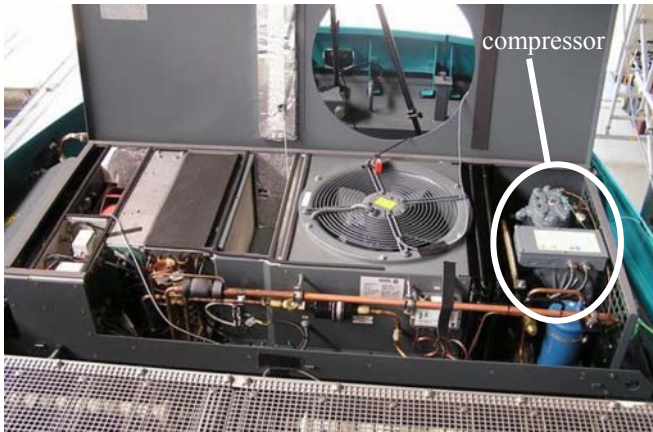
Fig. 1: General view of the HVAC unit mounted on top of a tram roof.
