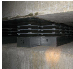
Figure 8 – Elastic bearings in position under dwellings on the pop centre during the construction phase
