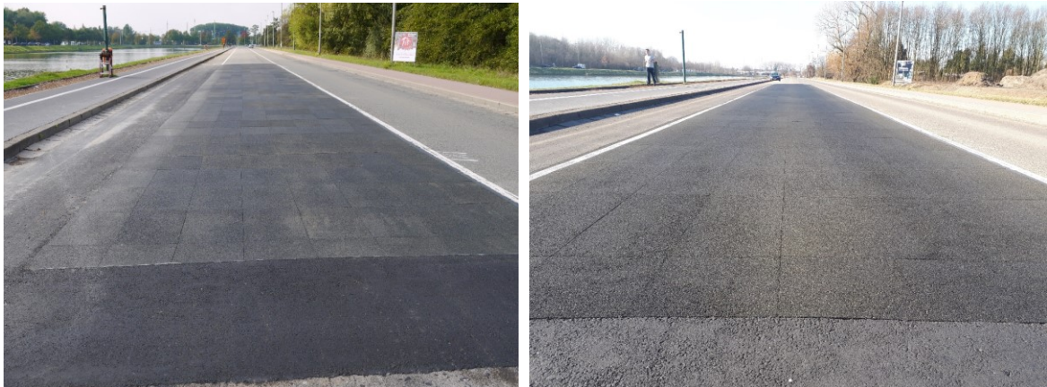
Figure 2 – The test track: on 8 October 2018, just after completion (left) and 4 months later, on 29 February 2019 (right). Some slight “general” raveling is noticeable.
