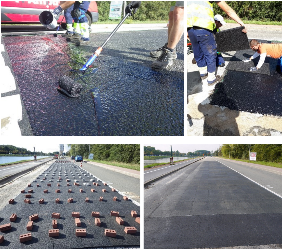
Figure 1 – The construction of the test track: spreading of the epoxy glue (upper left hand side), the placing of the slabs (upper right hand side), weights on the corners of the slabs during the drying of the glue (lower left hand side) and the finished test track (lower right hand side)
